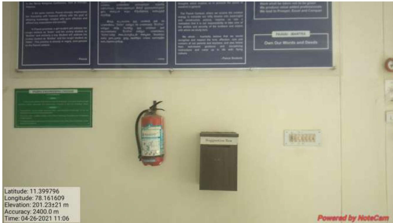
FIRE EXTINGUISHER NEAR TEMPLE TOWER LIFT
