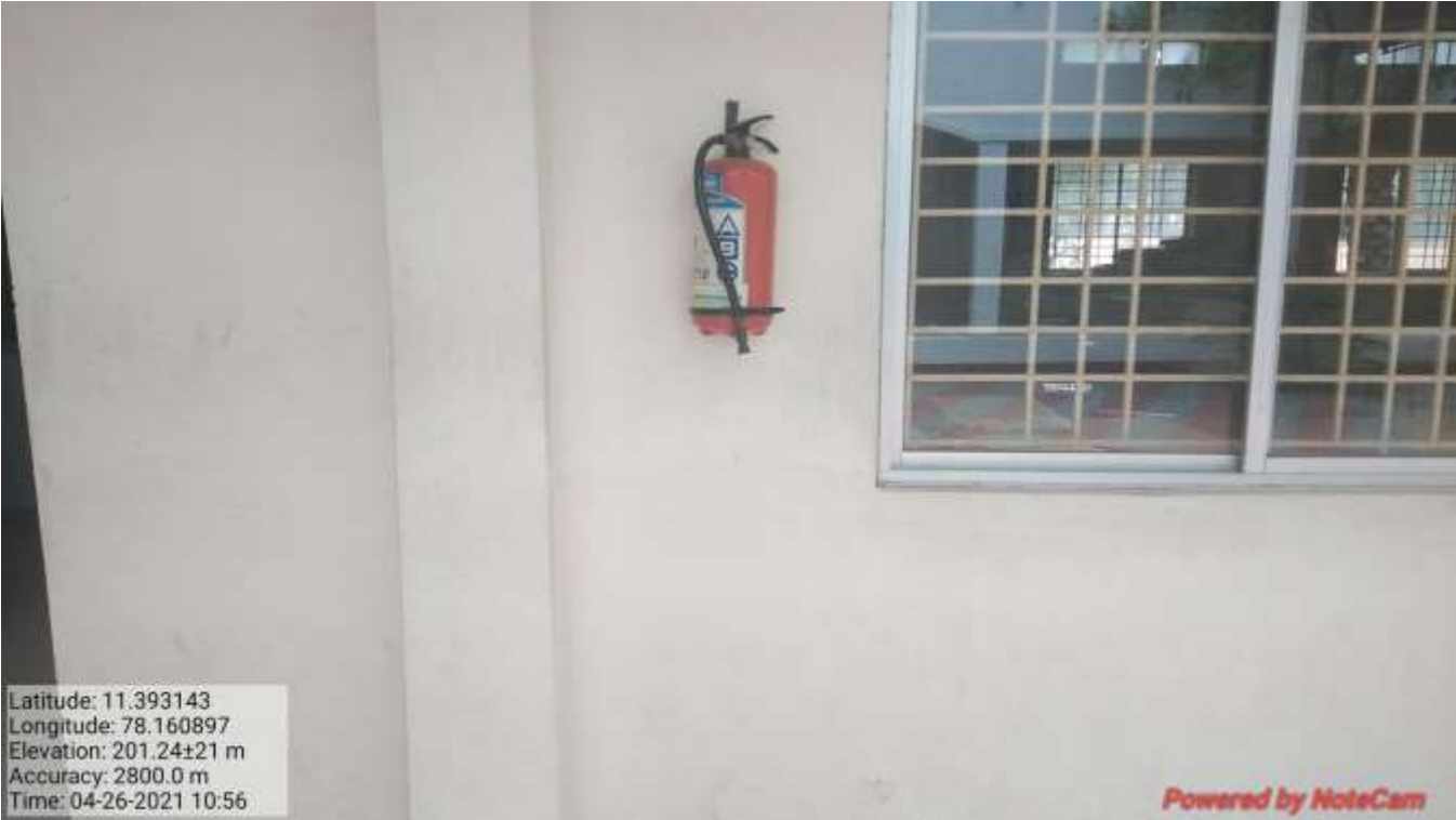
FIRE EXTINGUISHER NEAR CAD/CAM LAB
