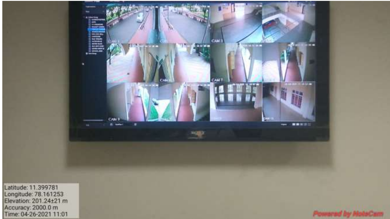
CCTV CAMERA DISPLAY
