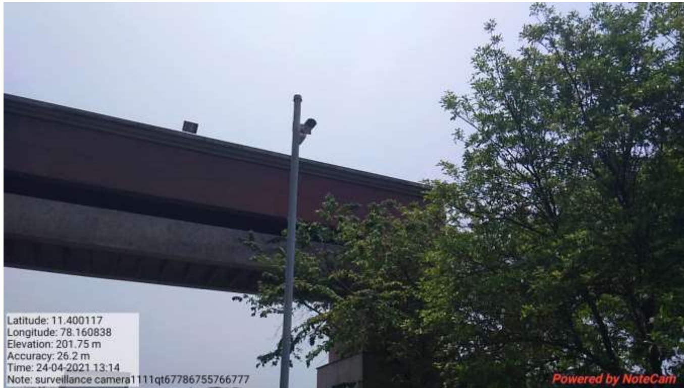
CCTV CAMERA NEAR LADIES HOSTEL
