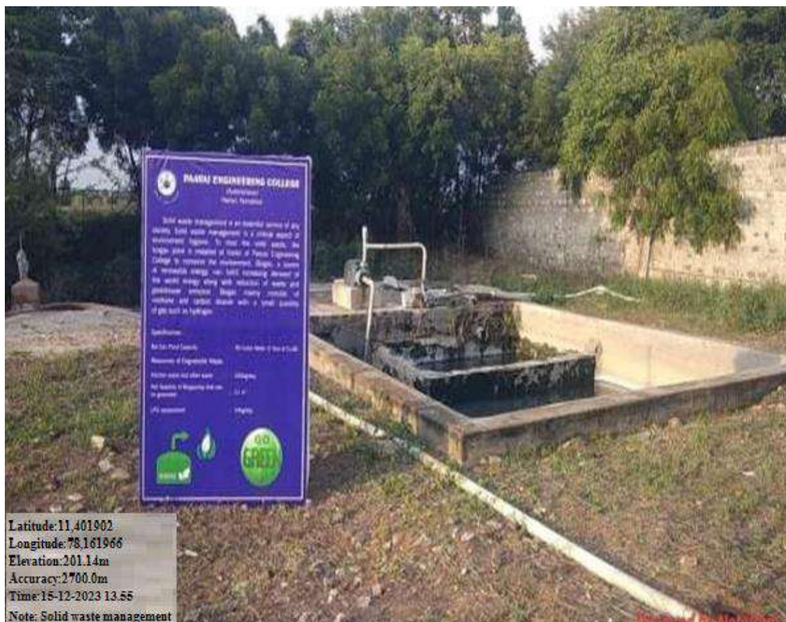
Fig: Biogas Plant
