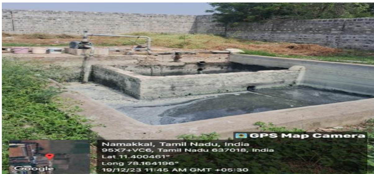
Fig: Biogas Plant
