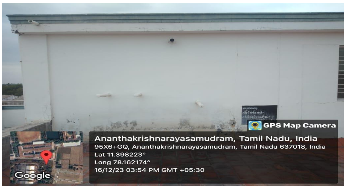
Water Tank 3 with capacity of 5,000 Litres
