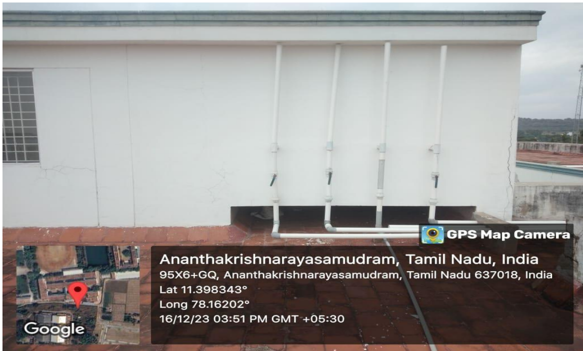
Water Tank 2 with capacity of 5,000 Litres
