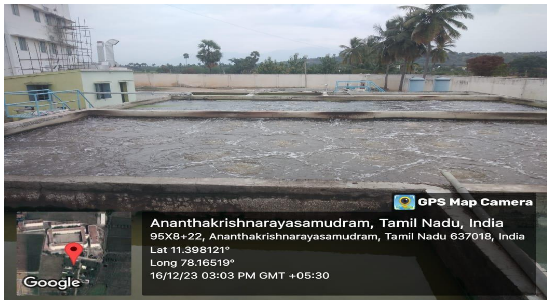
Waste Water Recycling plant
