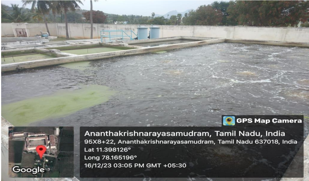
Waste Water Recycling plant
