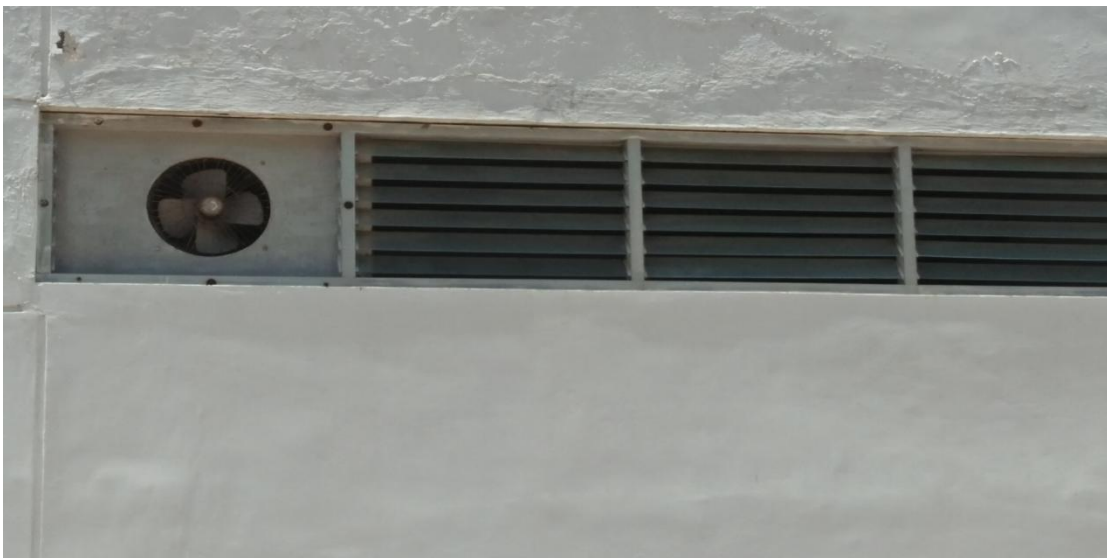
Fig.4. Exhaust fan located in the toilets
