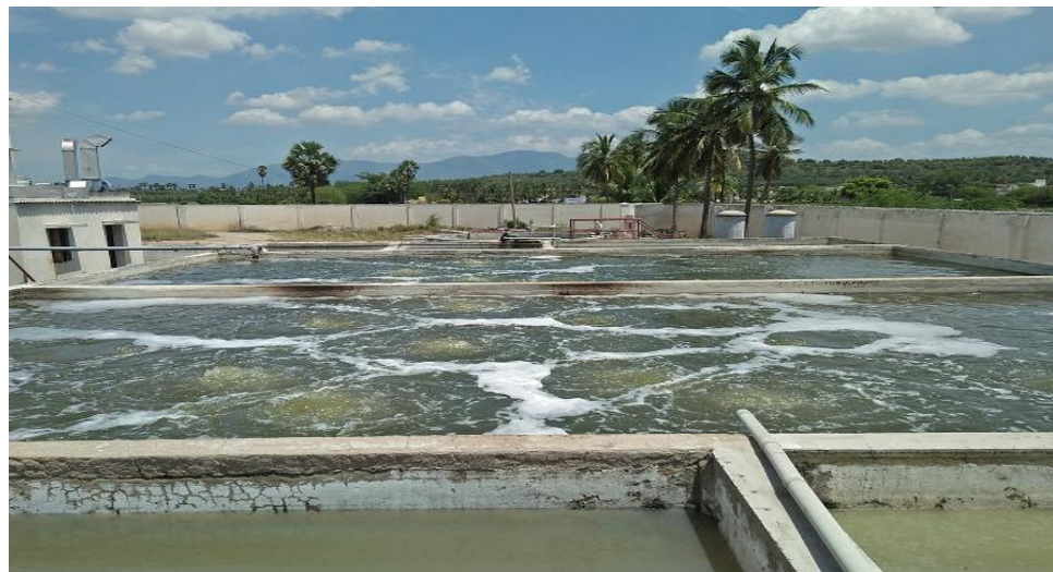
Fig.7. Water treatment plant
